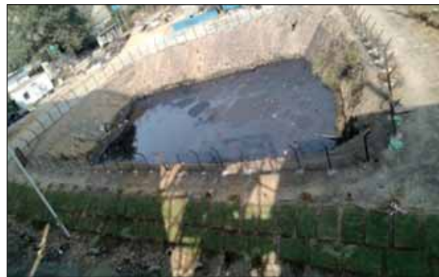
Fig. 6.3 : Catch pond for the plant drainage system
