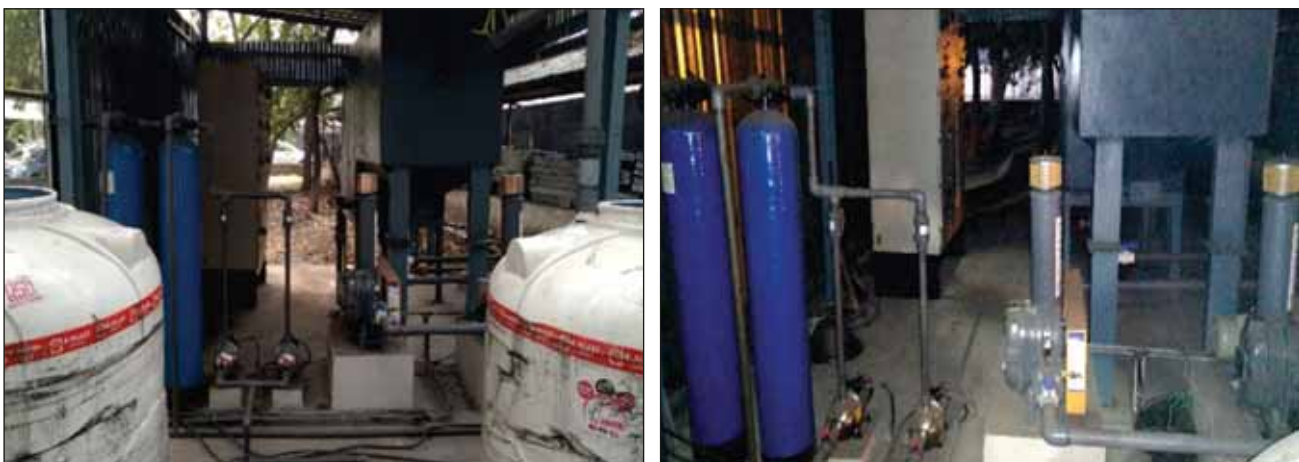
Pic. 6.4 : Effluent treatment plant
